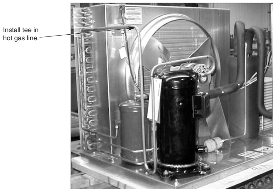
Figure 2 - Hot Gas Line
