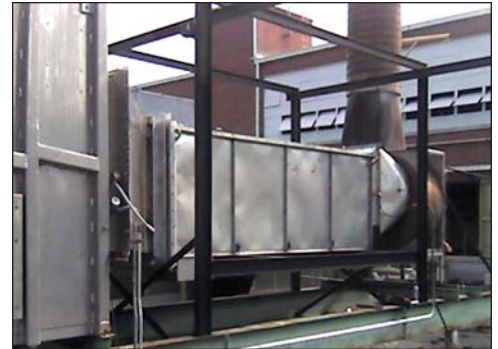
A Mueller model EB-XT Temp-Plate energy bank in use at the chemical plant.
