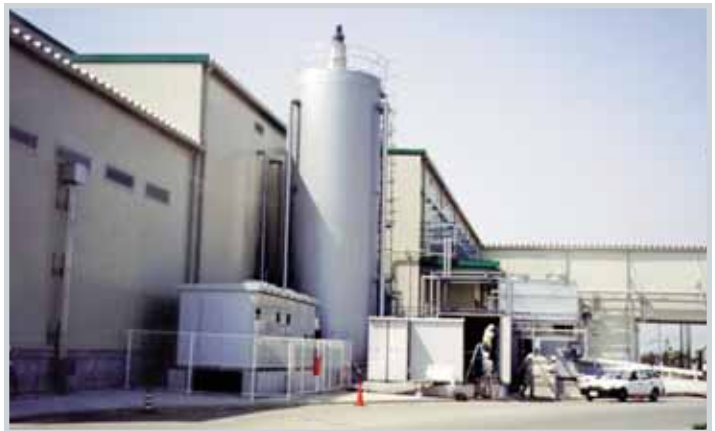
ORE-100 units installed at a dairy processing plant in Japan. The use of a silo ice-storage tank saves expensive land.
